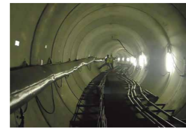
チリウン川工事推進管内 Inside pipes installed in the Ciliwung River Project
