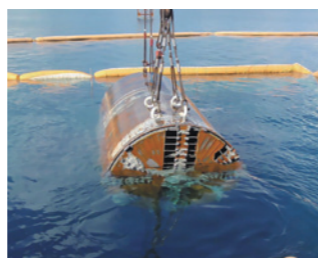
海中からの掘進機の回収 Collecting a tunneling machine from the ocean
