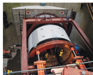
超大口径管の推進状況（発進立坑） The jacking method for the ultra-large diameter pipes is in process (starting shaft)
