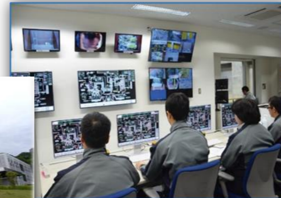
Operation and monitoring facilities
