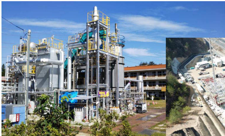
Biomass power plant (Furudono-town)
