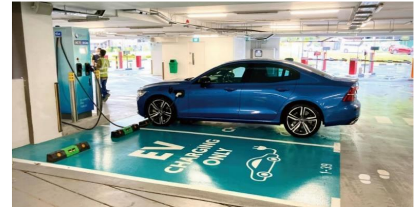
EV Charger Installation Work in Singapore (987 EV chargers to be installed at total of 314 sites)
