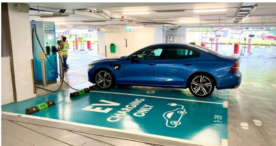
987 EV chargers to be installed at total of 314 sites
