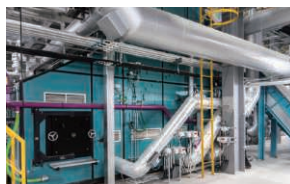
Biomass boiler in Ritto City
