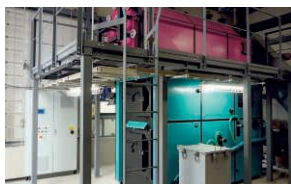
Biomass boiler in Hachimantai City
