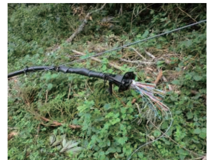
Cable cut by a fallen tree
