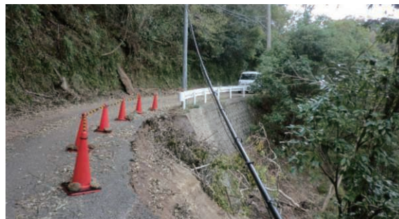
Downed utility poles and hanging cables due to landslide
