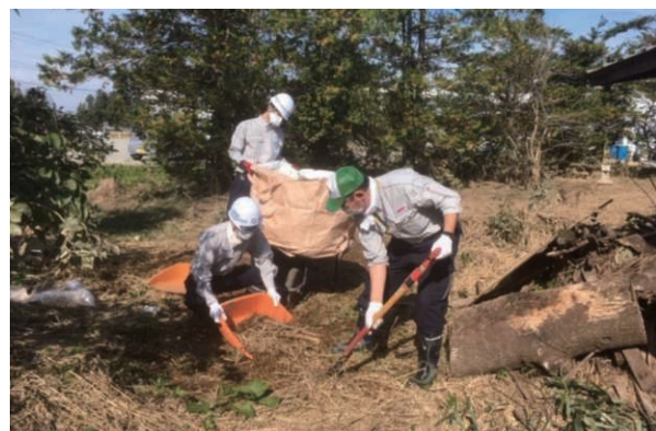
Removing rice straw washed ashore by a flood in front of the volunteer center
