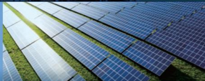
Solar power generation facilities
