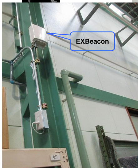
Photo of equipment introduced in Company A
