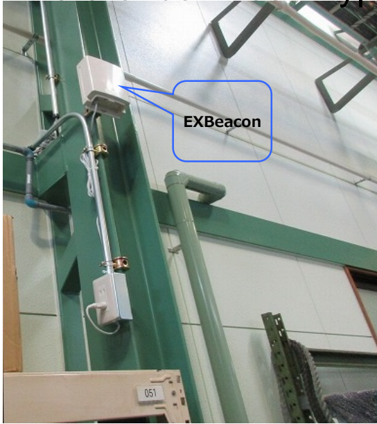
Photo of equipment introduced in Company A
